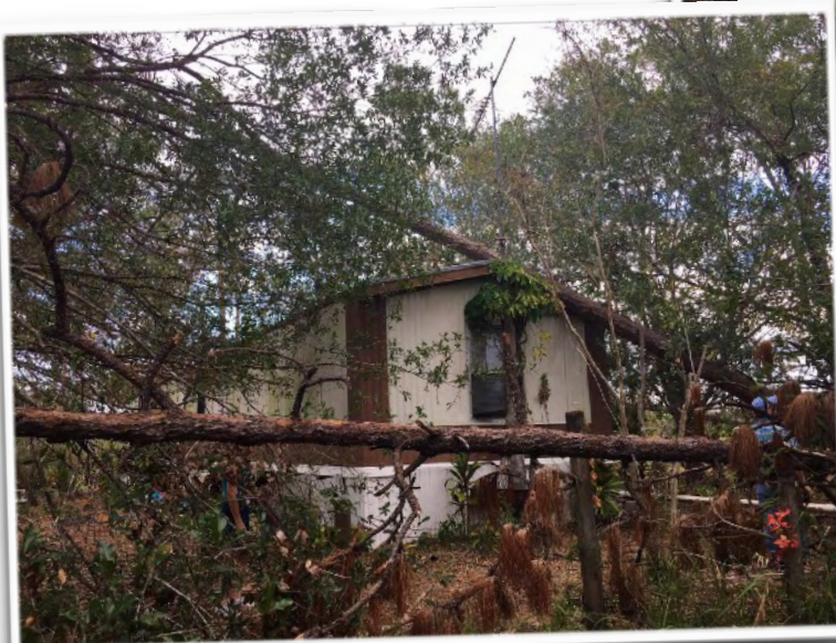
This home is in nearby Glades county where you can see the tree is still on the roof.
